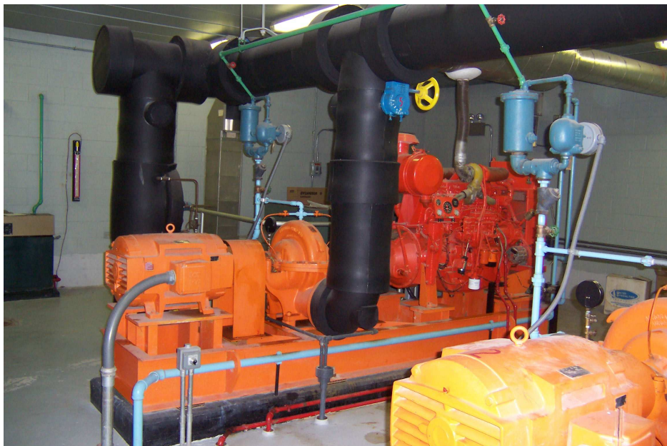
Booster Pump at Cornell
