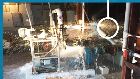
Broken fresh water feed
