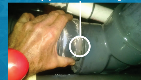
Broken pipe due to shifting
