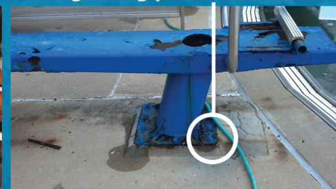
Rotting diving platform stanchion
